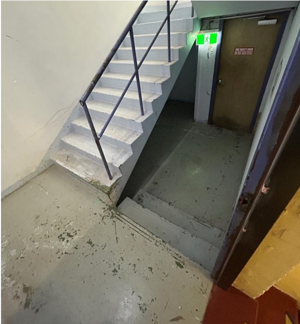
Figure 9: The fire exit located in the adjoining lot, which is accessible from the subject site and which exits on Grafton Lane. The fire exit is a registered easement for which the subject site benefits.
