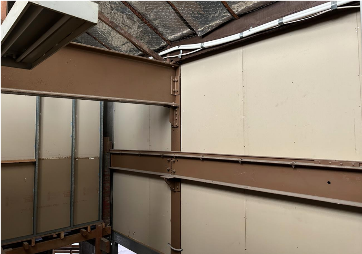
Figure 11: Interior with an example of the steel beams (upper beam) proposed to be retained, and a hoist beam (lower beam) to be removed
